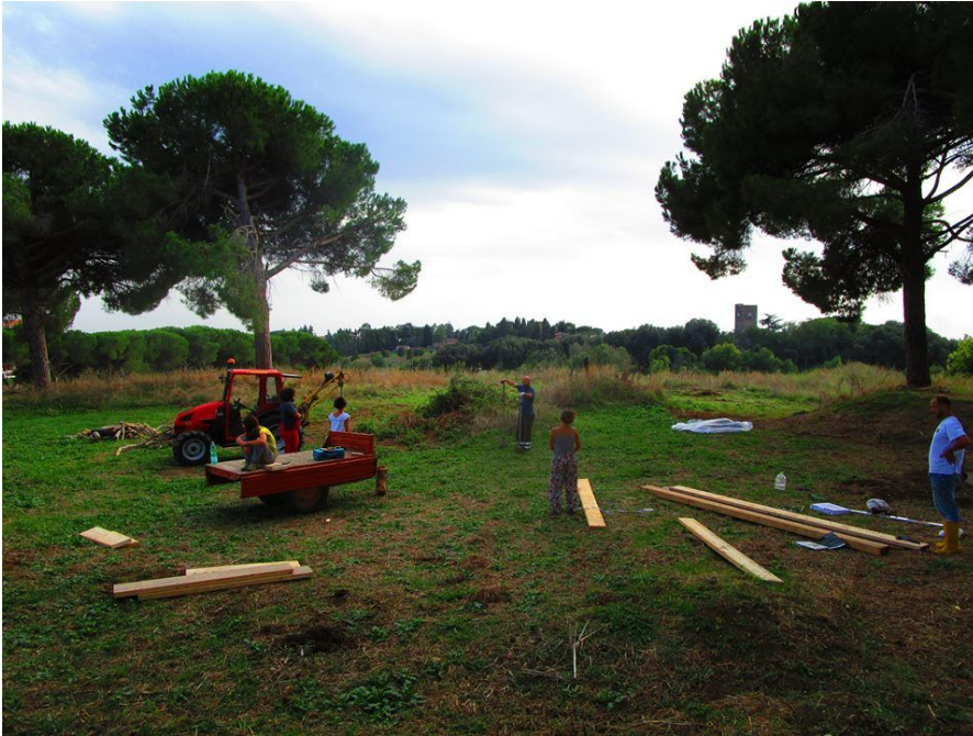
Figure 1: Borghetto San Carlo – work in progress (credit Giacomo Lepri, source: CoRAgGio: https://www.facebook.com/CoopCoraggio ).
